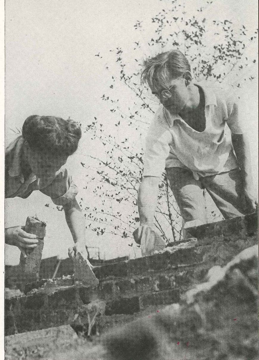
Work campers and members of the local community worked together to build Flanner House, Negro Community center in Indianapolis, Indiana
